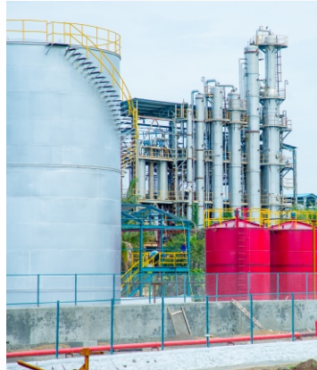
Ethanol Storage Tanks
